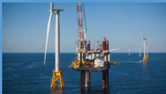
Construction on the Block Island Wind Farm finished this year. (Photo Credit: Deepwater Wind)
