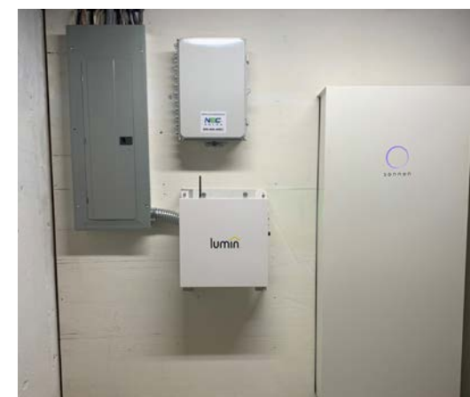
Many microgrids, such as those developed through the Resilient Microgrids for Critical Services Program, incorporate battery storage such as shown here (OER)
