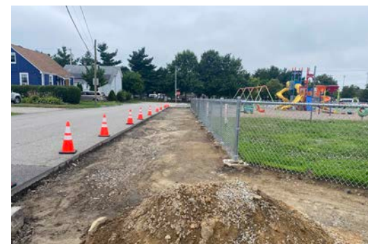
Impervious surface removal in preparation for green infrastructure and plantings at Agnes B Hennessey Elementary School, funded by EPA OSG Grants (RIIB)
