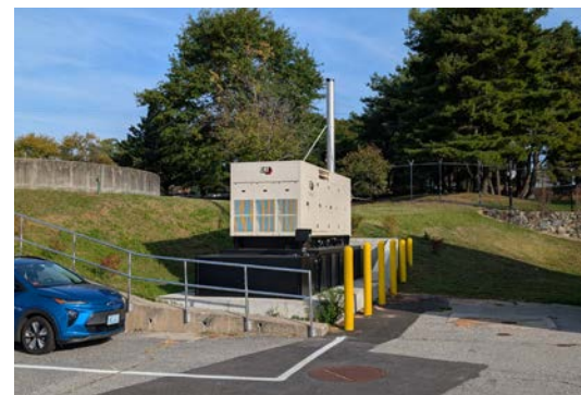
Floodproofing resiliency measures installed at the East Greenwich Wastewater Treatment Facility, funded by the Wastewater Treatment Facility Resilience Fund (RIDEM)
