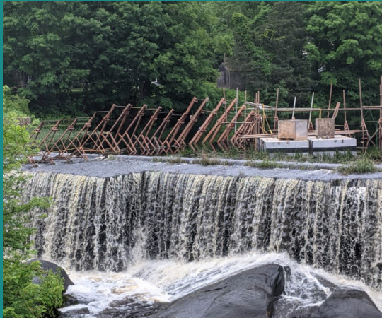
Repairs to the Wyoming Dam began in June 2021. Photo courtesy of RIDEM.
