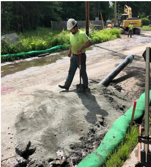
Slater'sville Public Supply Project - North Smithfield Drinking Water Main Extension. Photo courtesy of RIIB.
