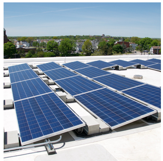
Solar installation on the Powers Building (RI Department of Administration). Photo courtesy of RI OER.
