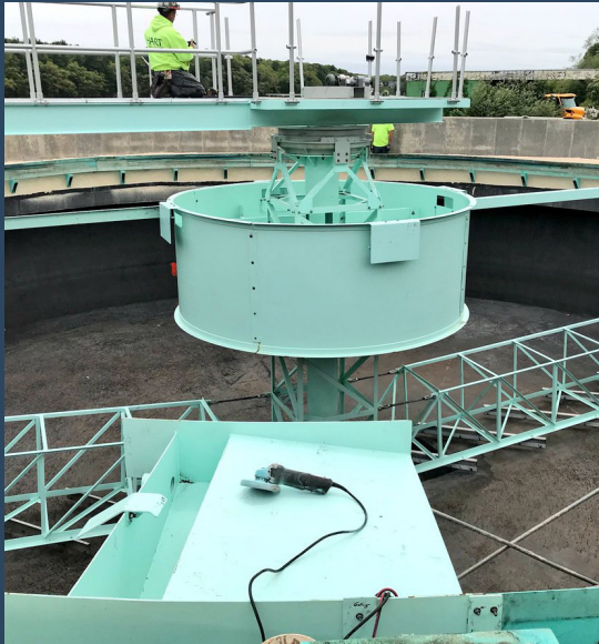
East Greenwich Wastewater Treatment Facility. Photo courtesy of RIIB.
