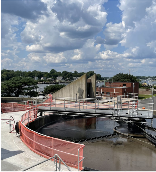
Warren Wastewater Treatment Facility - the first to incorporate flood protection measures identified in RIDEM's 2017 climate change vulnerability assessment. Photo courtesy of RIIB.
